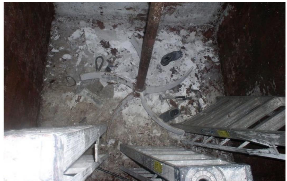
View of the bottom of the tank and the ladders used to enter and exit the tank.
