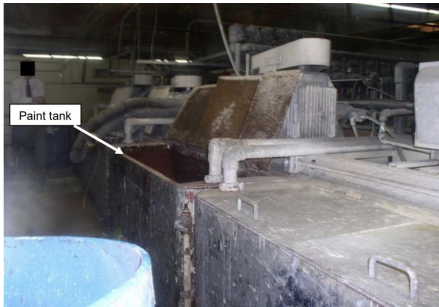
The paint tank being cleaned when this tragic incident occurred.
