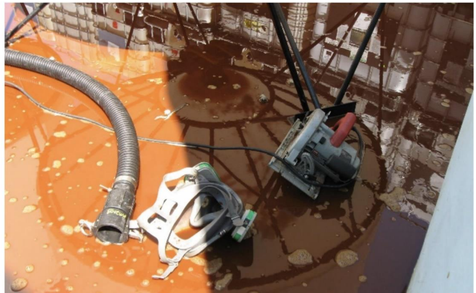
The bottom of the tank where the circular saw and the worker's respirator were left behind.
