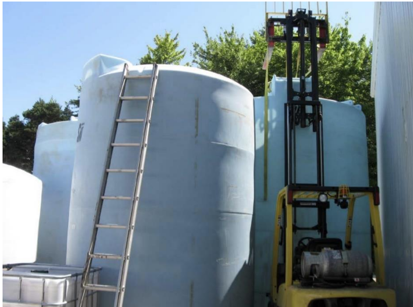
Tank where this incident occurred (back right) with the lift truck positioned in front of it.
