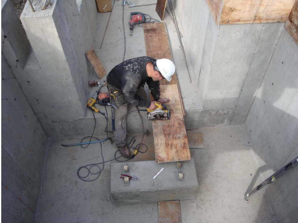
Working in a pit or confined area such the one in this photo could be dangerous if a generator or other smoke producing tools are used. (*3)
