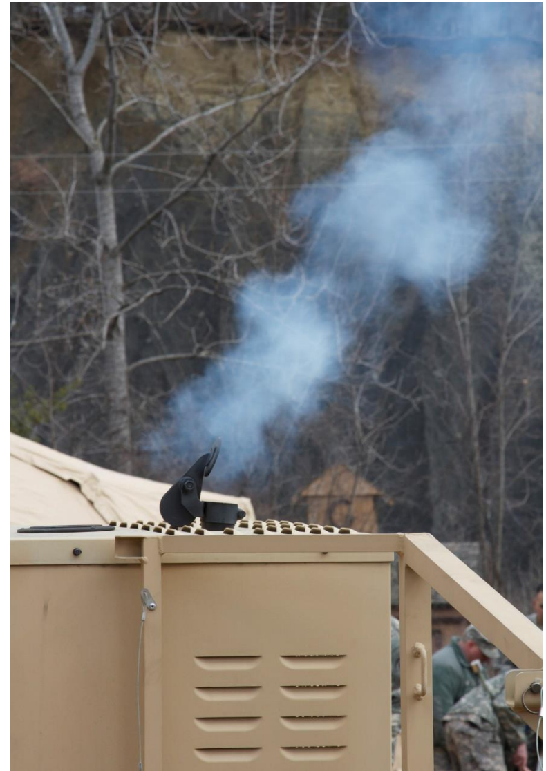
Image of smoke coming from a generator. High amounts of deadly CO gas could be found in this smoke. (*2)
