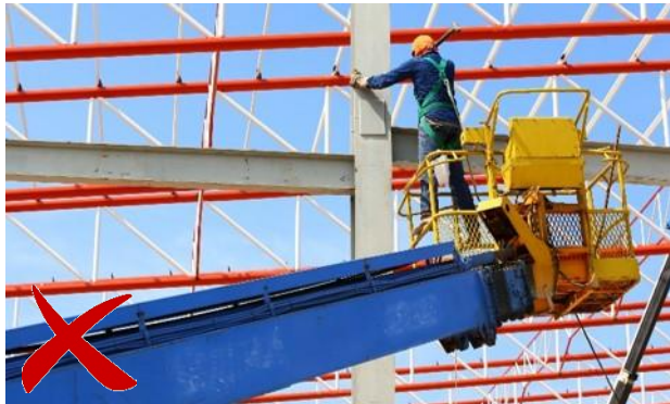
Never climb on guardrails.
