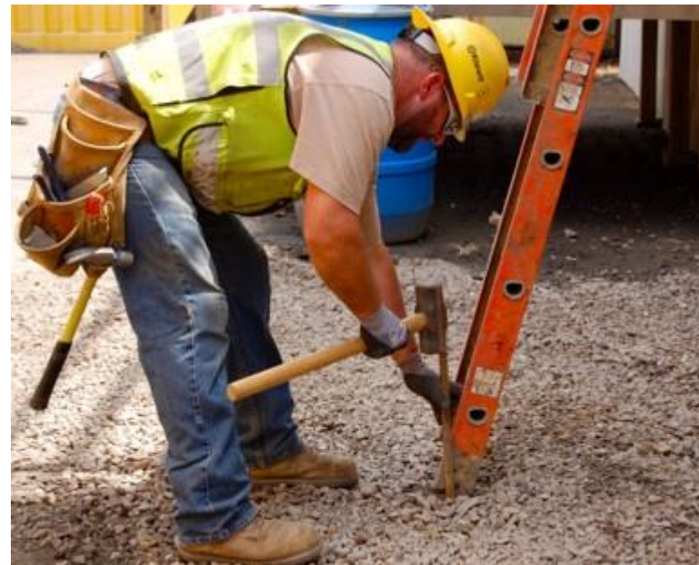
Staking and securing the side rails of a ladder to prevent falls. Image: Kiewit Power Constructors/eLCOSH.org
