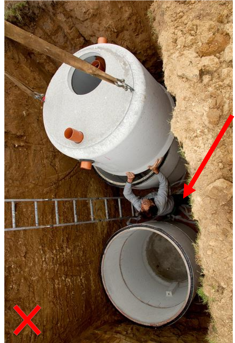
Man in unprotected excavation installing septic tank. Serious cave-in hazards exist in this situation. (*1)
