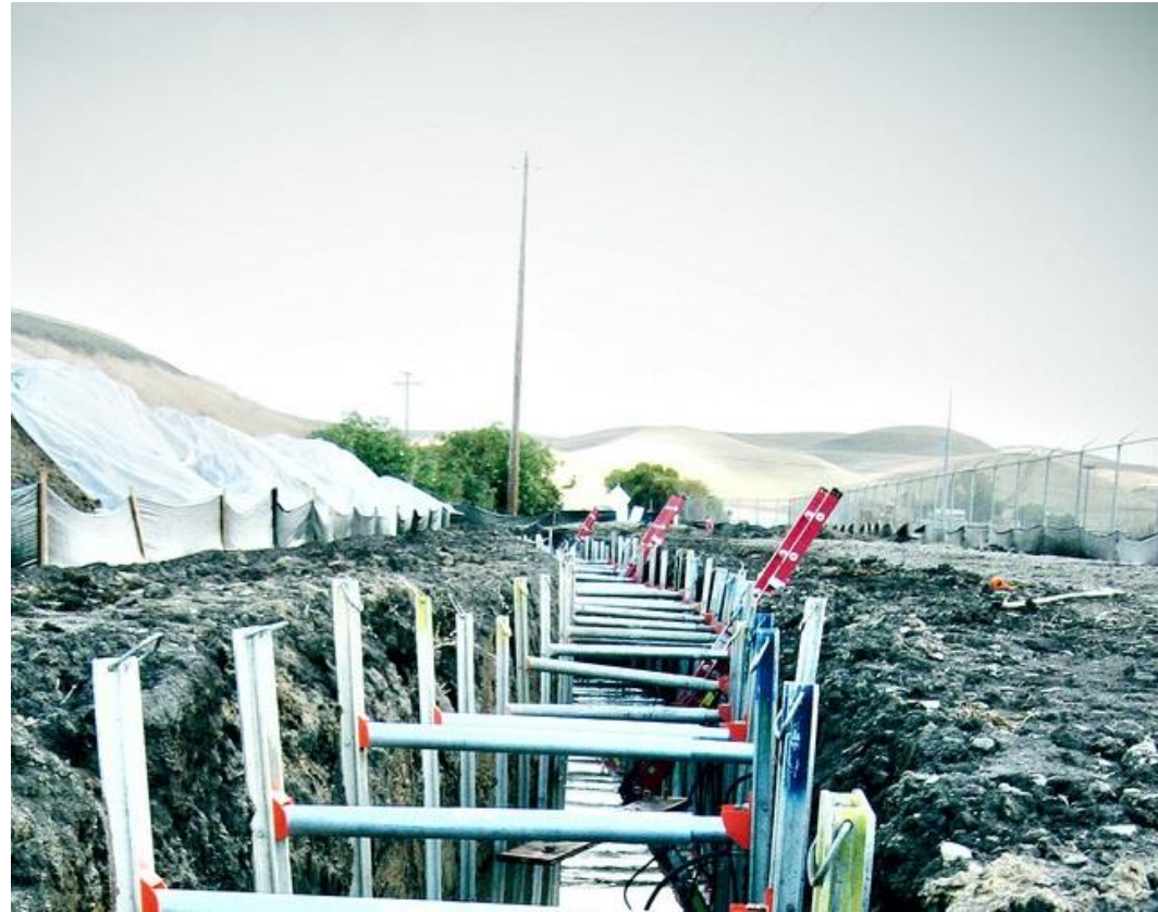
Hydraulic shoring system installed in this long trench. Note the ladders set up less than 25' apart and extending 3' above the excavation side as required by OSHA regulations. (*7)
