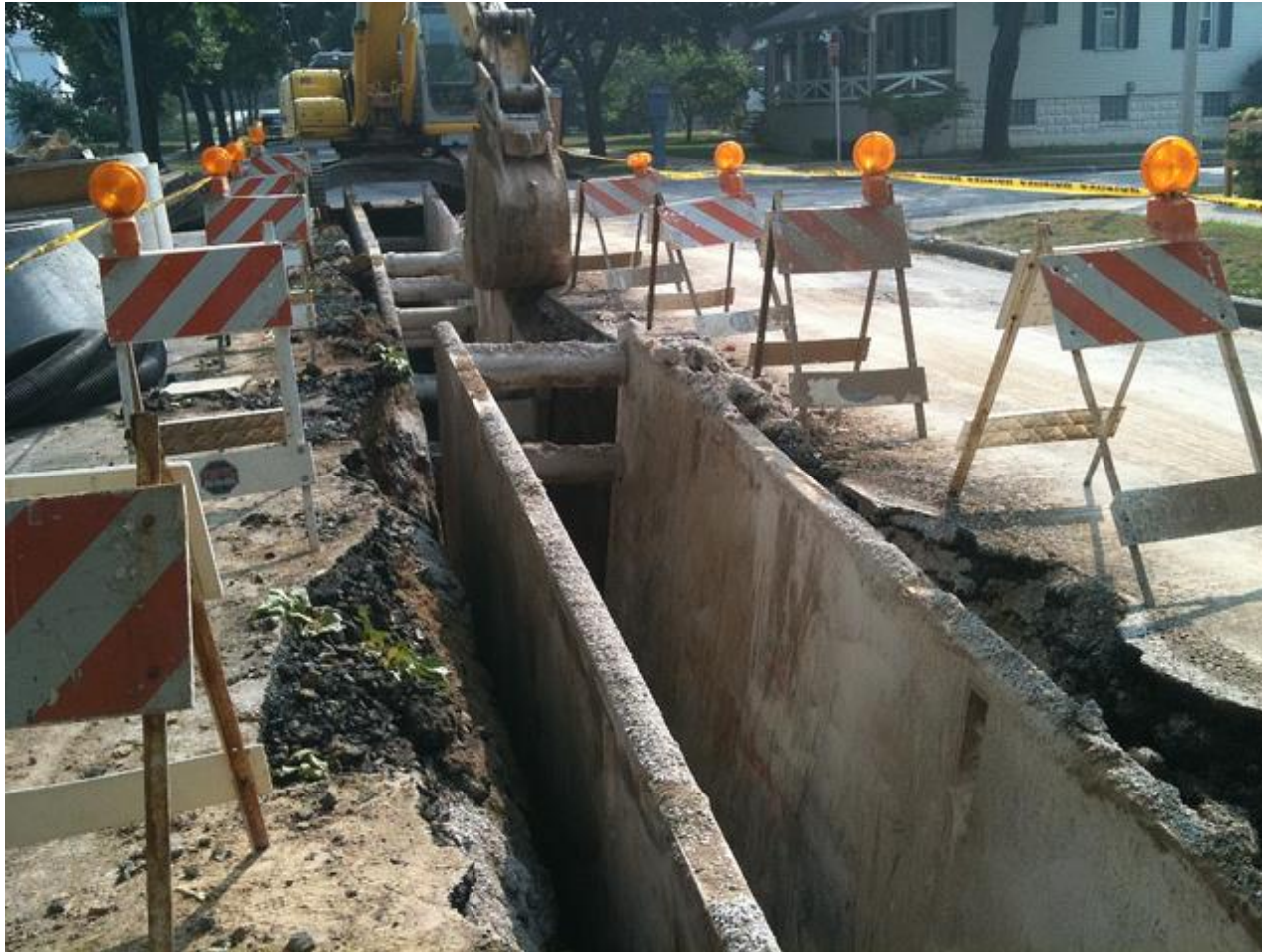
Example of trench boxes set inside of this excavation. Note that a ladder is not set up for safe entry at the time the photo was taken. (*6)
